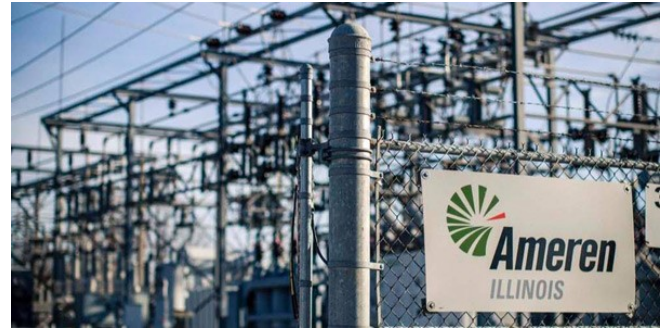
Ameren Illinois plans to file a petition with the Illinois Commerce Commission to be allowed to pass its tax-bill savings on to its electric customers. | Ameren Illinois
