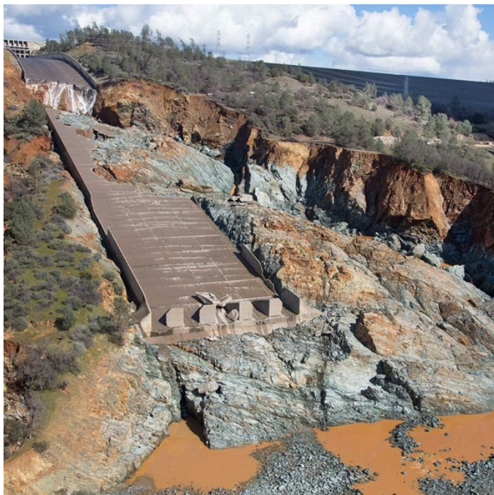
Damage to the Oroville Dam
